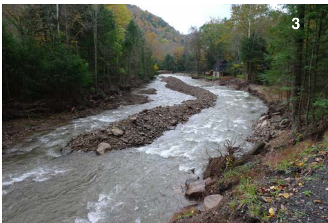
3. Removal of gravel point bar, realignment of main flow channel, regrading of channel slope and width. (late September 2011).
